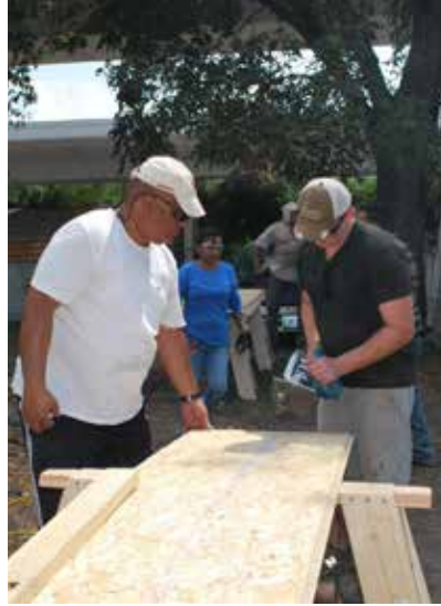
Construction technology students (top and bottom images) use skills to repair the home of an elderly couple.
